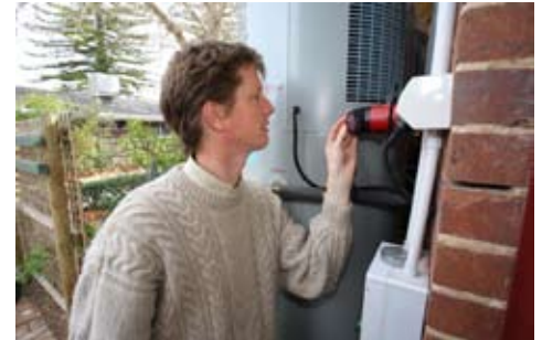
Chris monitoring the newly installed integrated hot water system and pressure pump.
